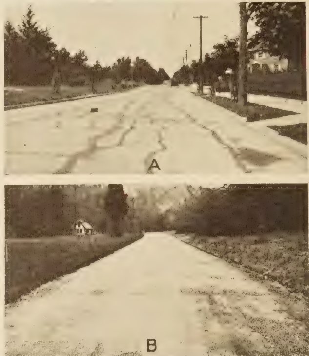
FIGURE 15.—DETRIMENTAL EFFECTS OF ELASTICITY OF SUBGRADE SOIL. A.—TYPE OF CRACKING LIKELY TO OCCUR IN PAVEMENTS LAID ON IMPROPERLY PREPARED ELASTIC SUBGRADES. NOTE CRACKS REFLECTING RUTS IN SUBGRADE. B.—ALLIGATOR HIDE CRACKING IN MACADAM ROAD SURFACE
